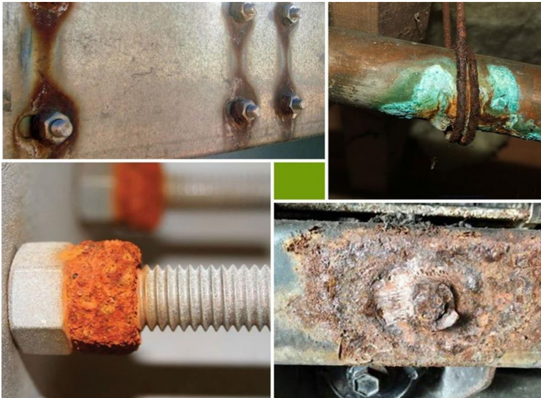
Figure I.6 : Electrochemical Corrosion (Galvanic Corrosion)
