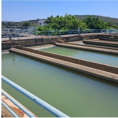
Figure 8: Bassin de filtration (Photo Hendi Fathi 2026)
